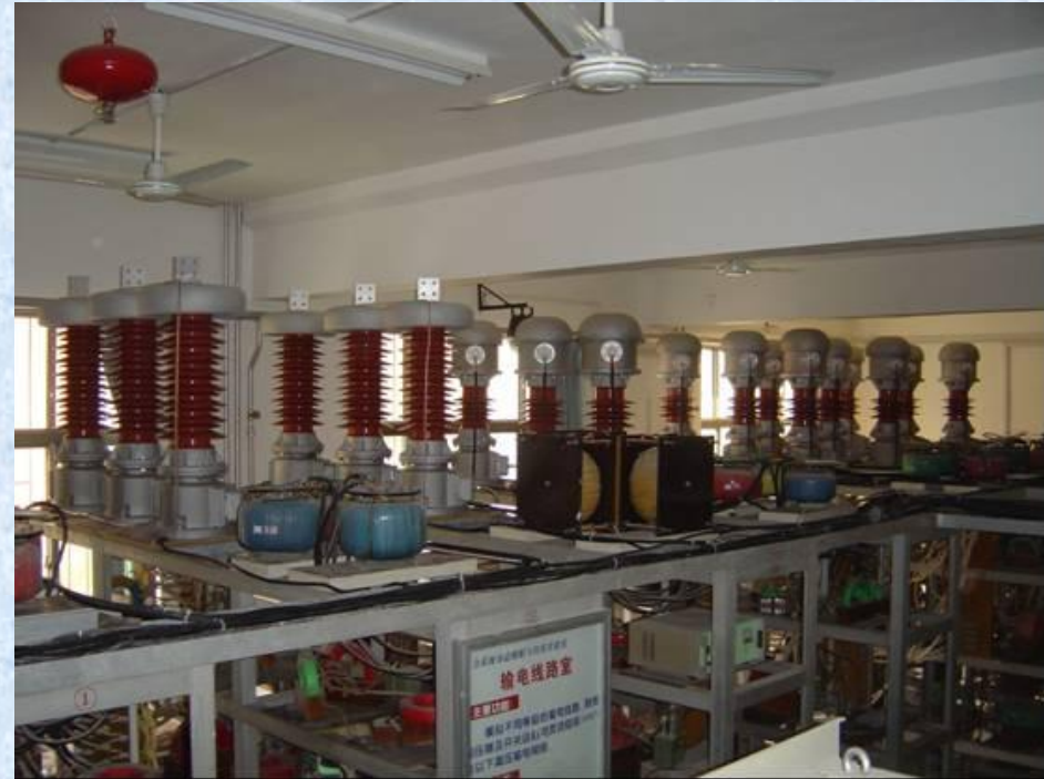
The installed ECTs and EVT
