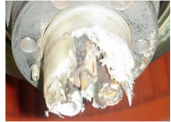
Rotor Lead Failure
