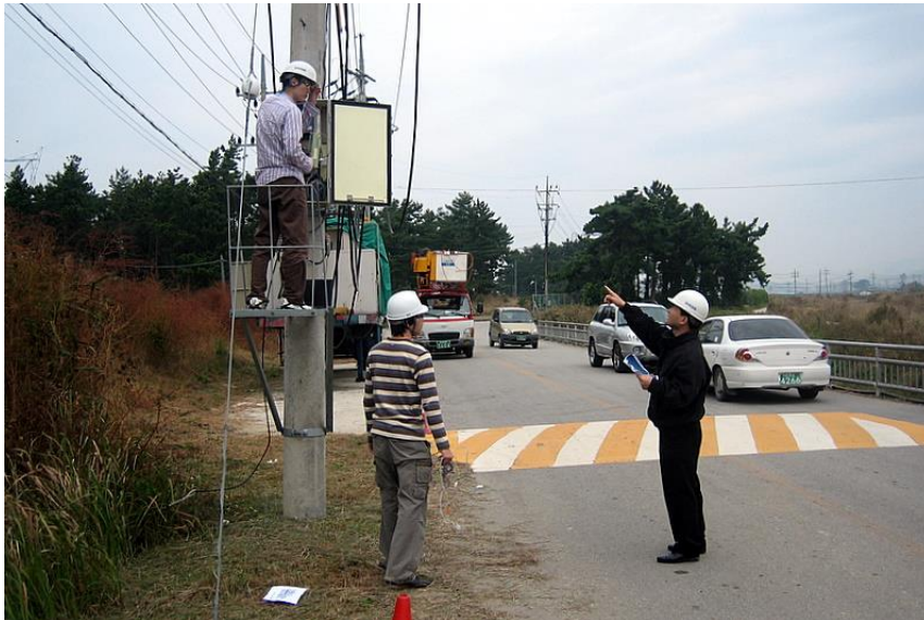
Gochang power test center in Korea (Preparing field test)
